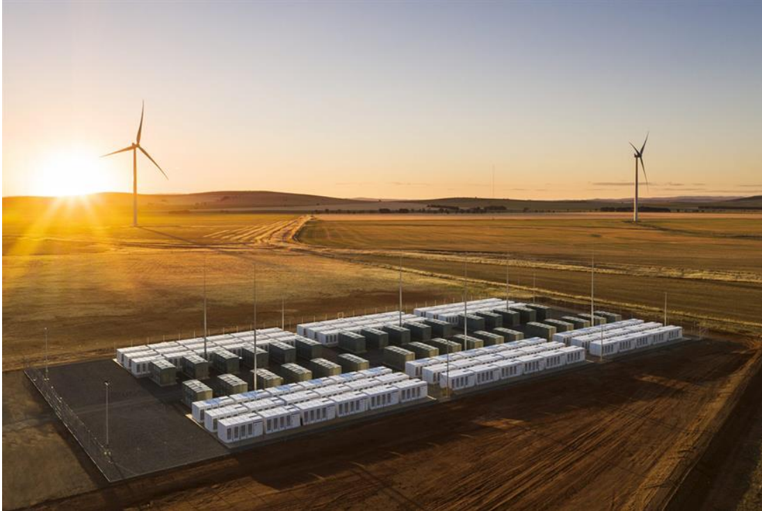
Hornsdale Battery Reserve – South Australia
