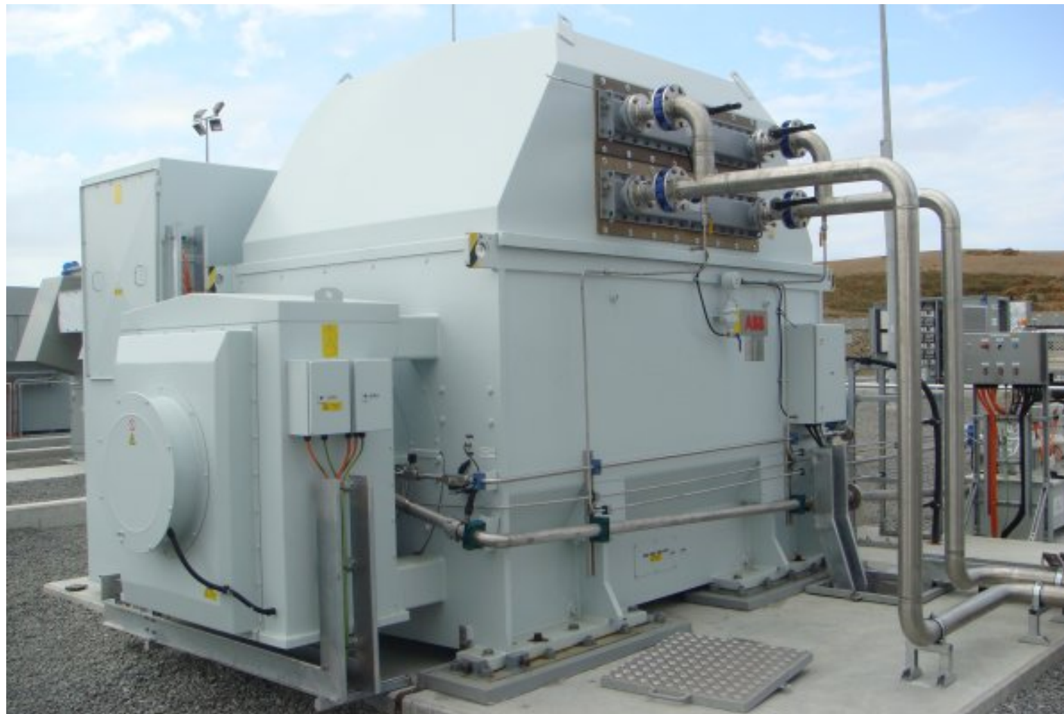
Hitachi ABB Synchronous Condenser
